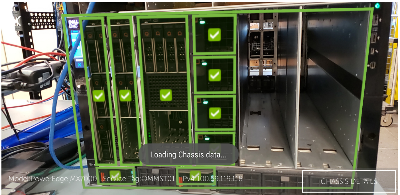
Figure 51. Monitor an MX7000 chassis by using AR
