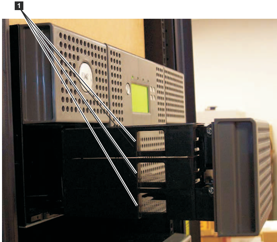
Figure 63. Finger Holes on back side of 4U library I/O station
