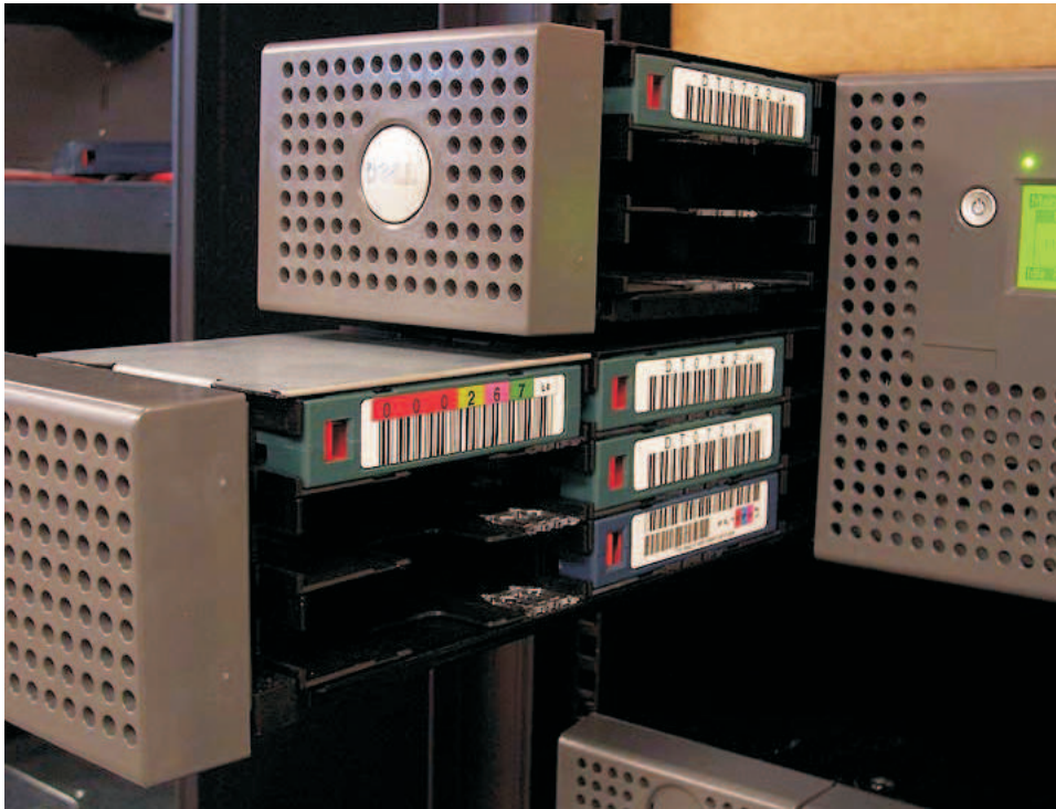
Figure 158. Left magazines pulled out of a 4U library (facing front of library)
