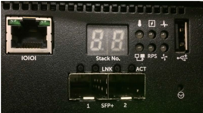
Figure 3-6. Dell Networking N2024 Close-up
